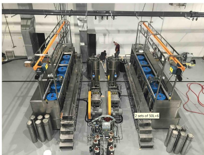
Photo 13 CO2 Extraction Unit
